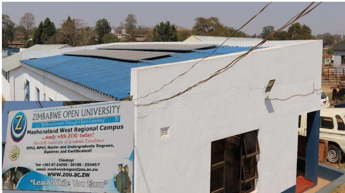
Rooftop view of the solar system
