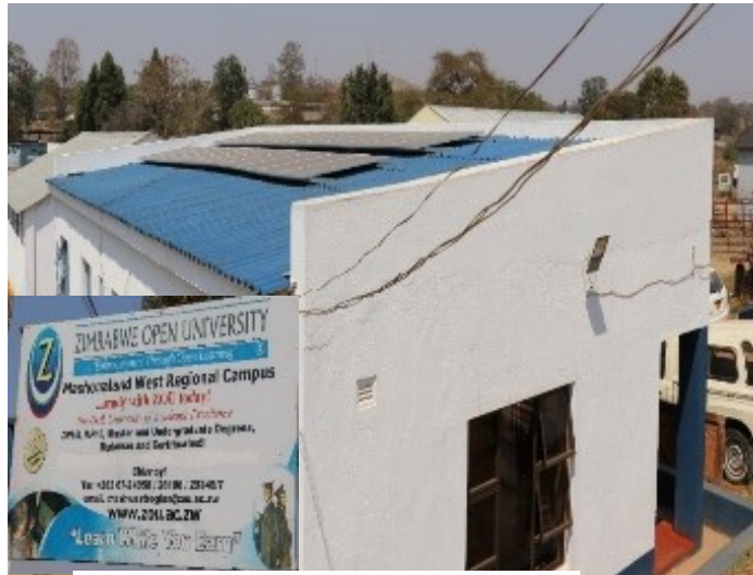
Roof top Solar panels at Mashonaland West Regional Campus
